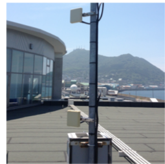
Fig. 4. Installation of antenna at Hakodate Research Center for Fisheries and Oceans (HRCFO).
