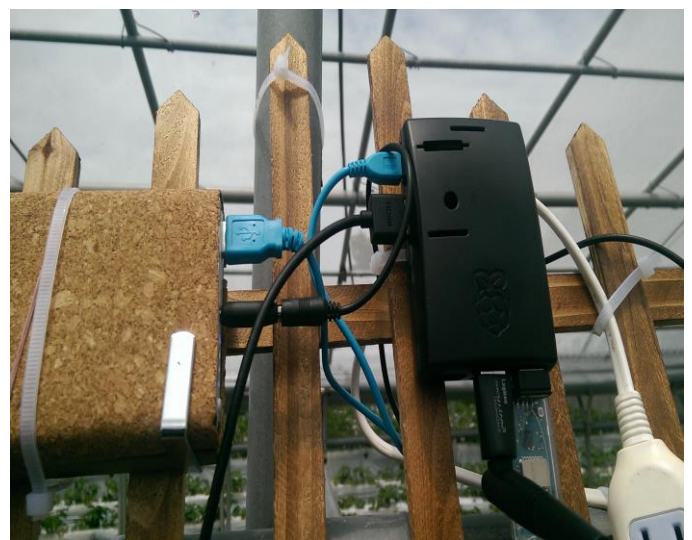
Figure 4. Raspberry Pi was installed in a house
