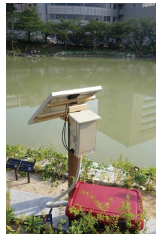
Figure 10. Gateway with Solar panel and Heavy duty battery
