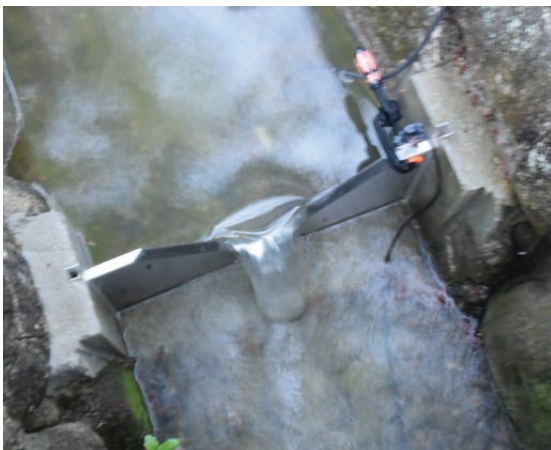
Figure 9. Overflowing after the heavy raifall at V-notch weir with eTape
