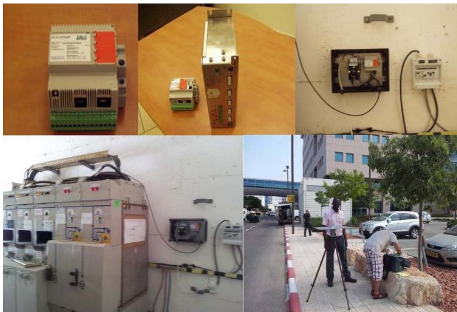
Figure 1: Modem Installations; Performance and EMC Measurements
