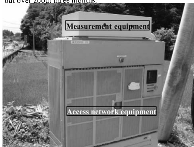
Fig.1 Access Network equipment
