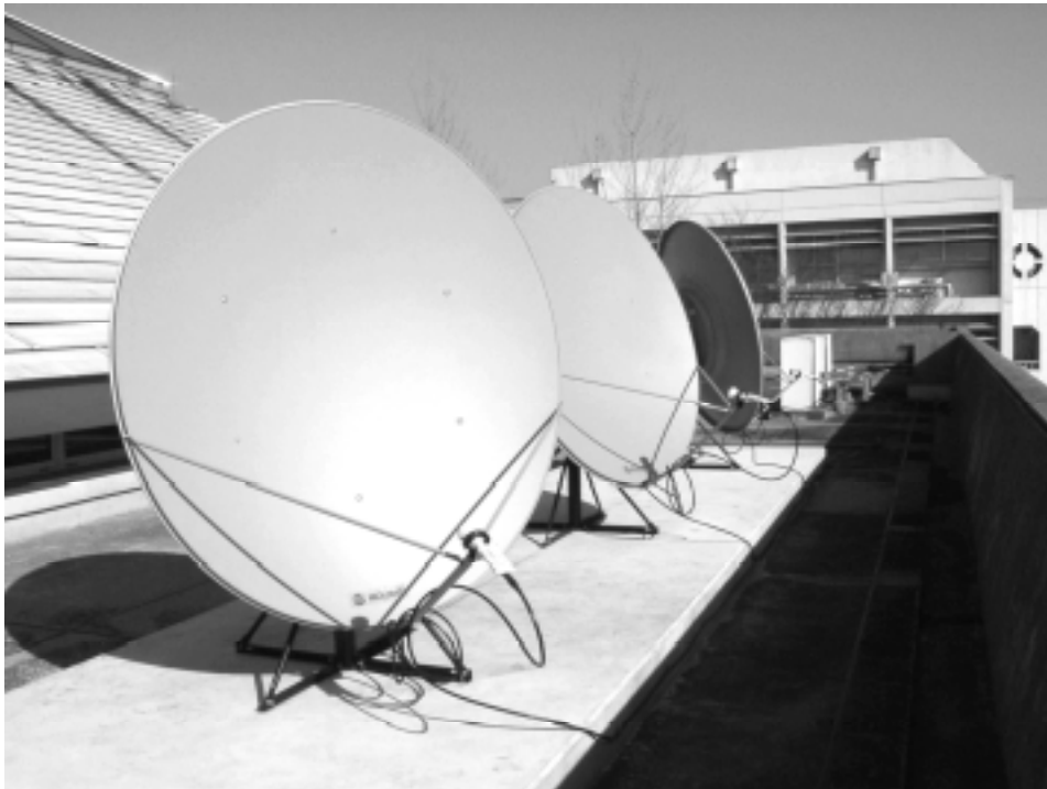
Figure 2. Ku-band receiving antennas for tomographic rain measurement system.
