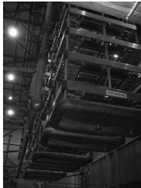
Fig. 3 Converter arrange in valve hall
