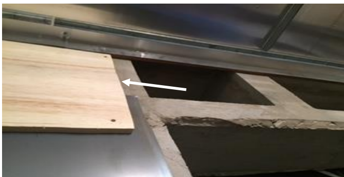
Fig. 2. Gap caused intentionally by the shield installer (white arrow).
