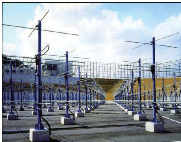
Fig. 2 Three-element crossed Yagi antennas of the MU radar
