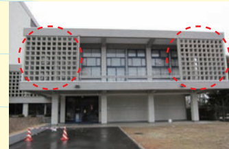
Tohoku University Centennial Hall is in danger of collapsing.
